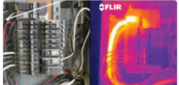
Hot Spot in an Electrical Panel
